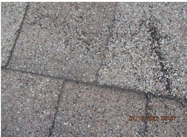
15. BUILDING NO. 14: TYPICAL GRANULE LOSS AND DETERIORATION OF SHINGLE
