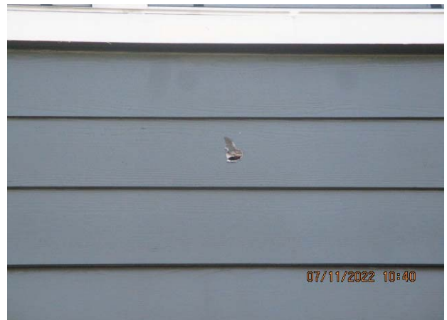
46. BUILDING NO. 21: PUNCTURE IN FIBER CEMENT SIDING
