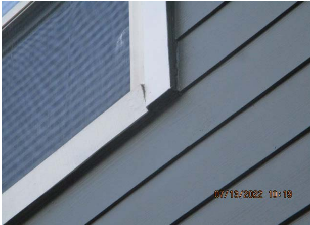
43. BUILDING NO. 6: TYPICAL DISPLACED FIBER CEMENT TRIM BELOW WINDOW SILL
