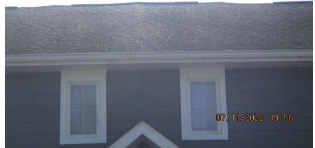
20. BUILDING NO. 21: FIBERGLASS REINFORCEMENT EXPOSED AT SHINGLE EDGES (NOTE SHINEY SPOTS)
