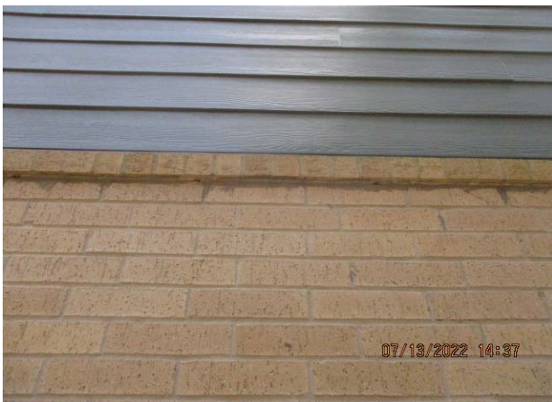
59. BUILDING NO. 19: TYPICAL REPAIR OF CRACK BETWEEN ROWLOCK BRICKS AND MASONRY VENEER
