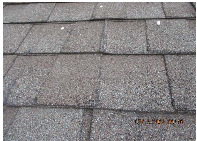
16. BUILDING NO. 14: TYPICAL GRANULE LOSS AND DETERIORATION OF SHINGLE
