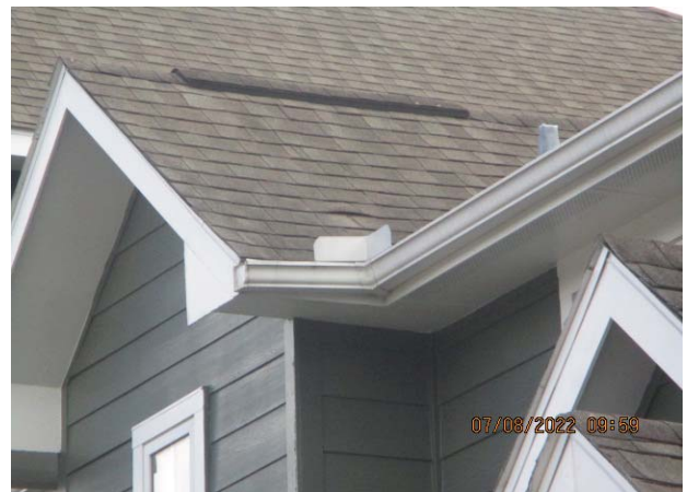
22. BUILDING NO. 15: BUCKLE IN SHINGLE
