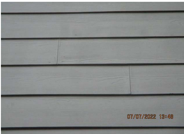
39. BUILDING NO. 14: SEALANT SPLIT AT BUTT JOINTS IN FIBER CEMENT SIDING
