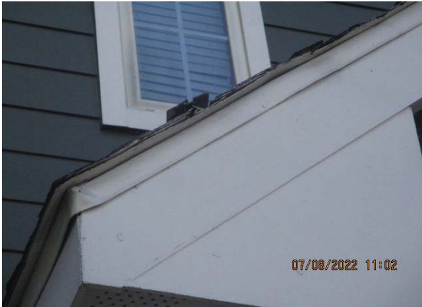
19. BUILDING NO. 15: TYPICAL DAMAGED SHINGLES AT RAKE EDGE
