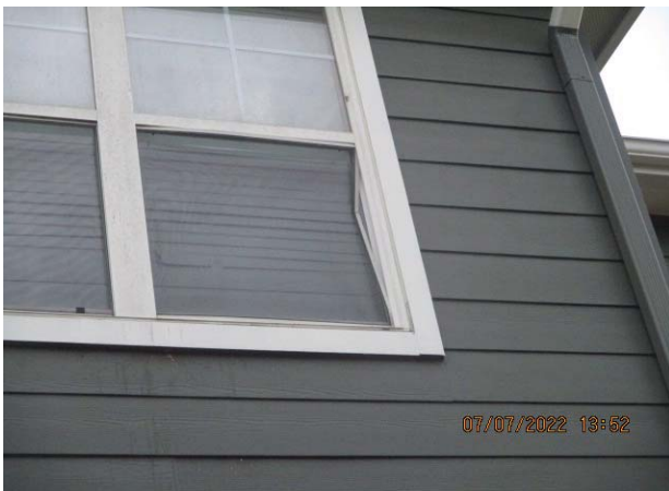
57. BUILDING NO. 13: TYPICAL DAMAGED SCREEN
