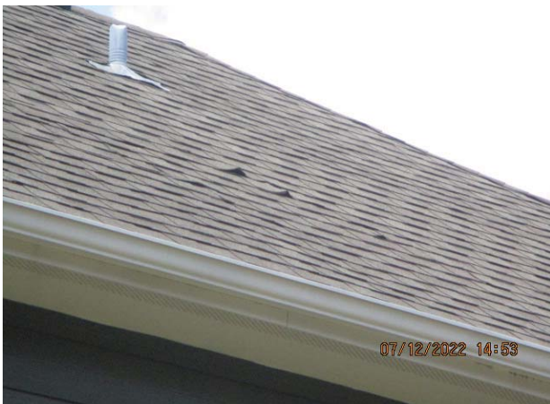
21. BUILDING NO. 9: BUCKLES IN SHINGLES
