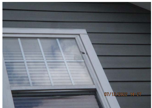
54. BUILDNG NO. 5: PUNCTURE IN VINYL WINDOW FRAME
