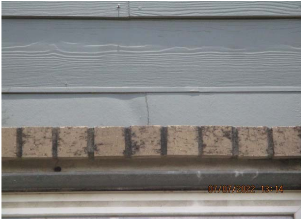
37. BUILDING NO. 14: TYPICAL CRACK IN FIBER CEMENT TRIM
