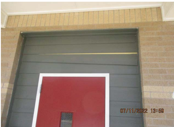
41. BUILDING NO. 24: LOOSE PIECE OF FIBER CEMENT SIDING
