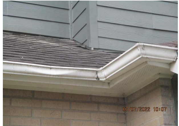
26. BUILDING NO. 14: SHINGLES RAISED UP OVER SHEET METAL RAKE FLASHING; NOTE BENT GUTTER
