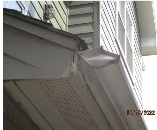
32. BUILDING NO. 22: GUTTER PARTIALLY PULLED AWAY FROM FASCIA
