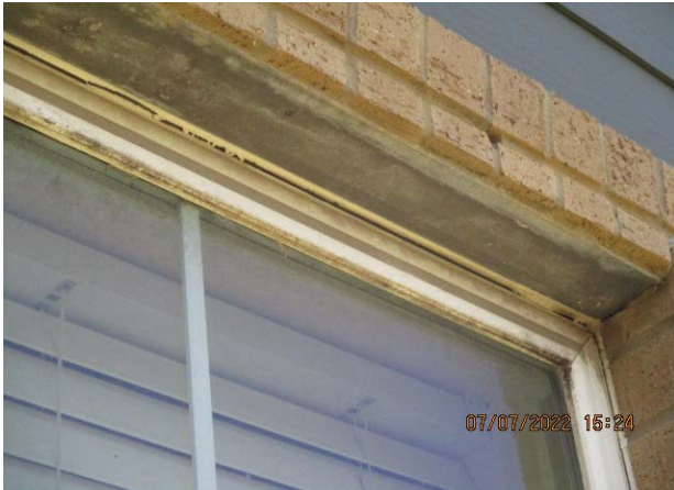
49. BUILDING NO. 16: TYPICAL DETERIORATED SEALANT AROUND WINDOW PERIMETER
