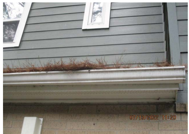
36. BUILDING NO. 22: PINE NEEDLE ACCUMULATION IN GUTTER
