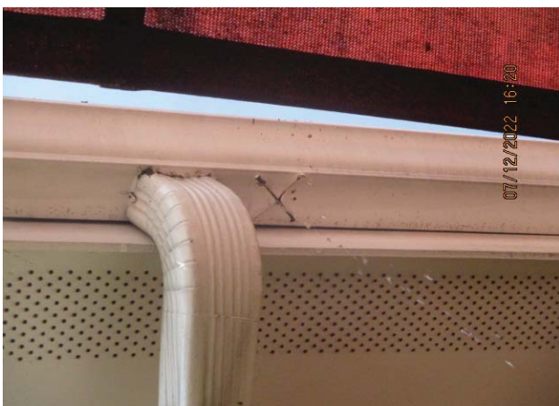
35. BUILDING NO. 2: UNSEALED CUT IN GUTTER FOR DOWNSPOUT
