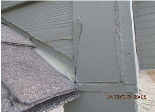
25. BUILDING NO. 14 CONTINUOUS SHEET METAL FLASHING AT RAKE CONDITION - NOTE GAP AT END OF METAL FLASHING
