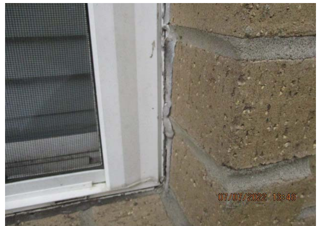
48. BUILDING NO. 13: TYPICAL DETERIORATED SEALANT AROUND WINDOW FRAME
