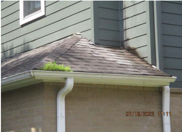
13. BUILDING NO. 22: TYPICAL SHINGLE REPAIR; NOTE VEGETATION GROWTH IN GUTTER
