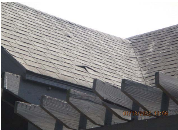
23. CANOPY: BUCKLES IN SHINGLES
