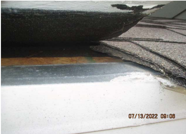
31. BUILDING NO. 14: UNDERLAYMENT DOES NOT EXTEND OVER FLANGE OF METAL DRIP EDGE AT EAVE
