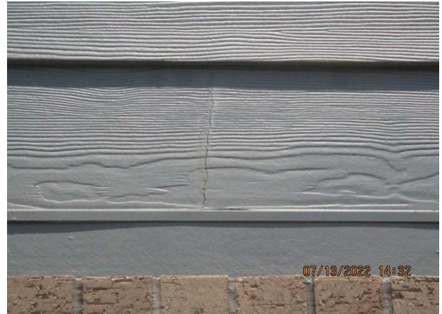
38. BUILDING NO. 20: TYPICAL CRACK IN FIBER CEMENT SIDING
