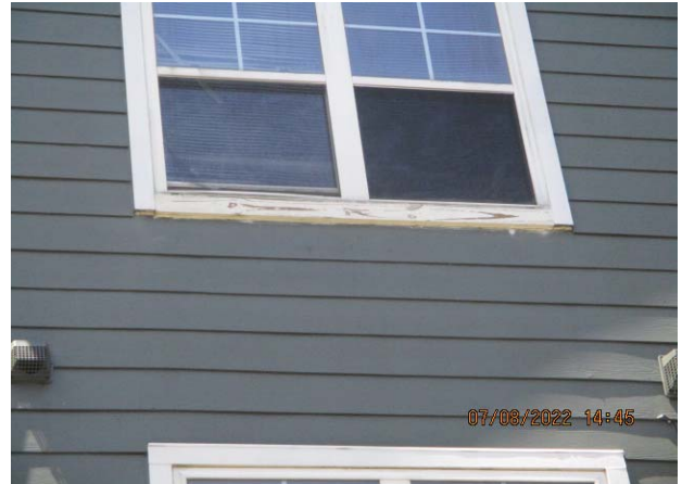
44. BUILDING NO. 18: PAINTED WOOD TRIM INSTALLED IN PLACE OF FIBER CEMENT TRIM
