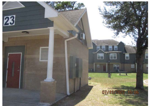
34. BUILDING NO. 23: DOWNSPOUT NOT ATTACHED TO GUTTER
