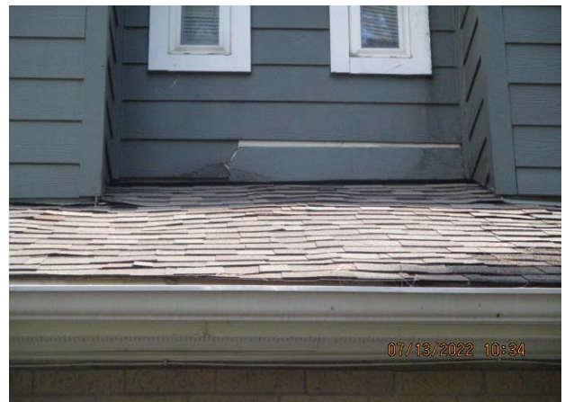
40. BUILDING NO. 6: LOOSE PIECE OF FIBER CEMENT SIDING
