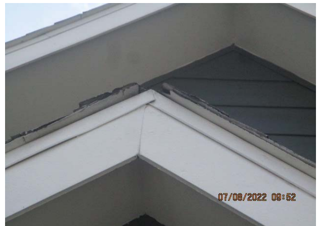
18. BUILDING NO. 15: TYPICAL DAMAGED SHINGLES AT RAKE EDGE
