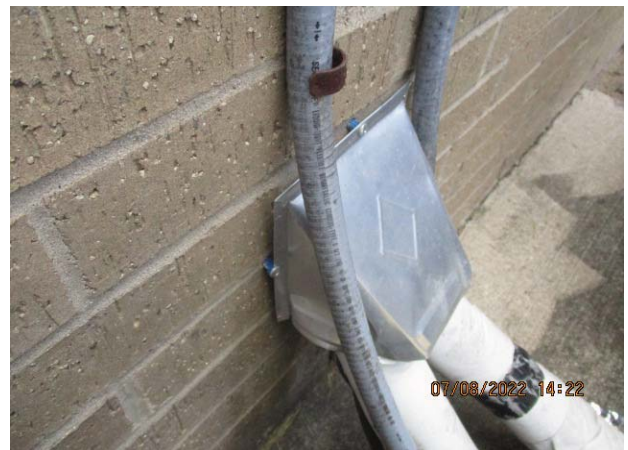
58. BUILDING NO. 18: TYPICAL UNSEALED HOOD OVER HVAC LINE PENETRATION
