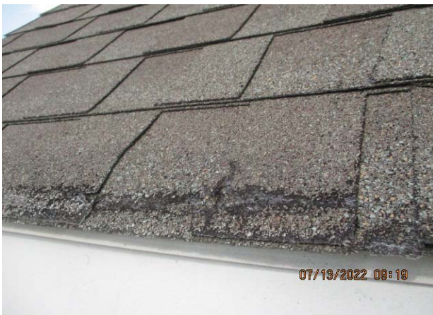
17. BUILDING NO. 14: TYPICAL DAMAGED SHINGLES AT LOW EAVE
