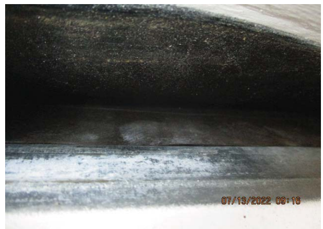
30. BUILDING NO. 14: UNDERLAYMENT DOES NOT EXTEND UNDER RAKE EDGE METAL DRIP EDGE
