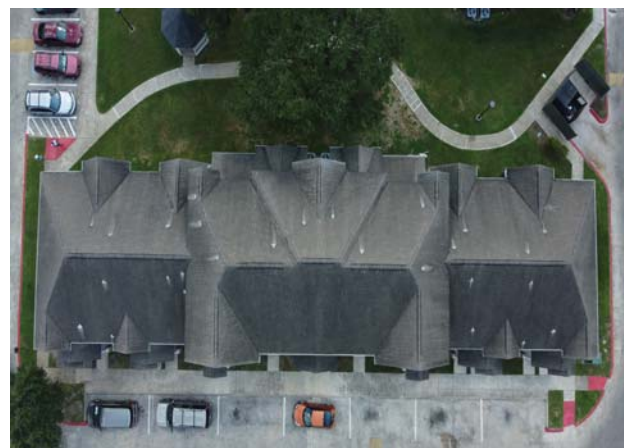
24. BUILDING NO. 16: OVERALL VIEW - NOTE DAMAGED RIDGE SHINGLES AND ROOF REPAIRS
