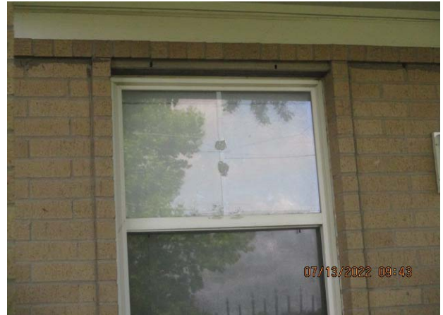
56. BUILDING NO. 12: BROKEN INSULATED GLASS LITE
