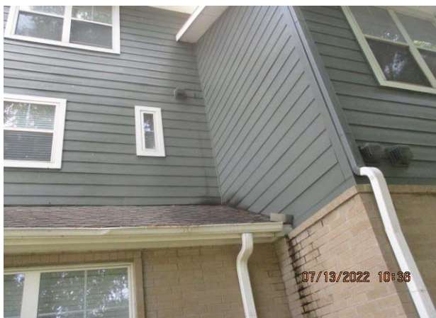
27. BUILDING NO. 6: CONDENSATE PAN OVERFLOW DRAIN LINE DRIPS ONTO ROOF AND SIDING
