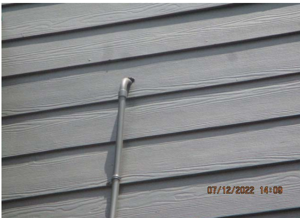
47. BUILDING NO. 3: TYPICAL UNSEALED CONDUIT PENETRATION
