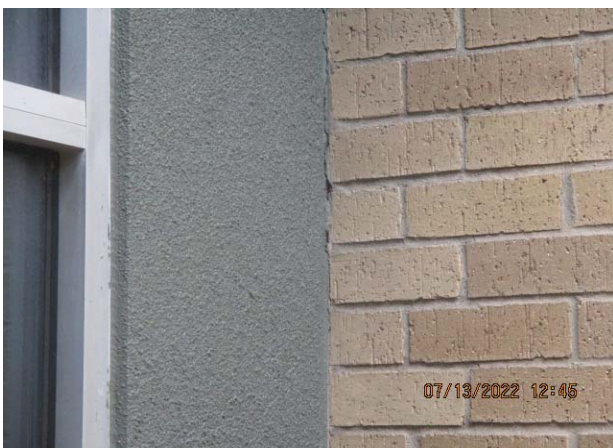
53. BUILDING NO. 1: UNSEALED JOINT BETWEEN PLASTER AND BRICK
