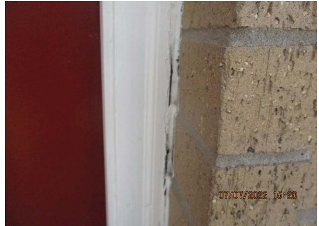
50. BUILDING NO. 16: SPLIT IN SEALANT AROUND DOOR FRAME
