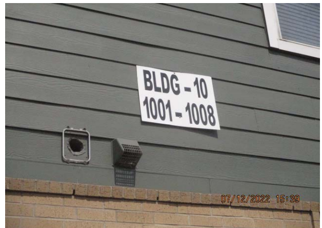
60. BUILDING NO. 10: TYPICAL MISSING DRYER VENT
