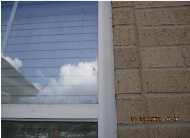
55. BUILDING NO. 15: BROKEN INSULATED GLASS LITE
