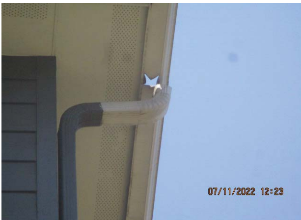
33. BUILDING NO. 4: DOWNSPOUT NOT ATTACHED TO GUTTER
