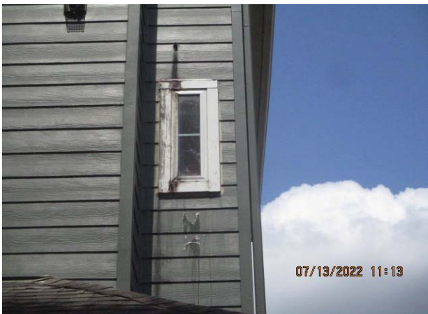
45. BUILDING NO. 22: DETERIORATED FIBER CEMENT TRIM; NOTE DRAINAGE FROM CONDENSATE OVERFLOW DRAIN
