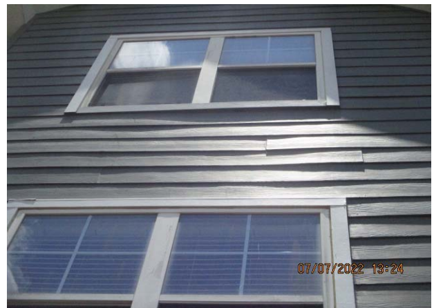
42. BUILDING NO. 13: TYPICAL WARPED FIBER CEMENT SIDING
