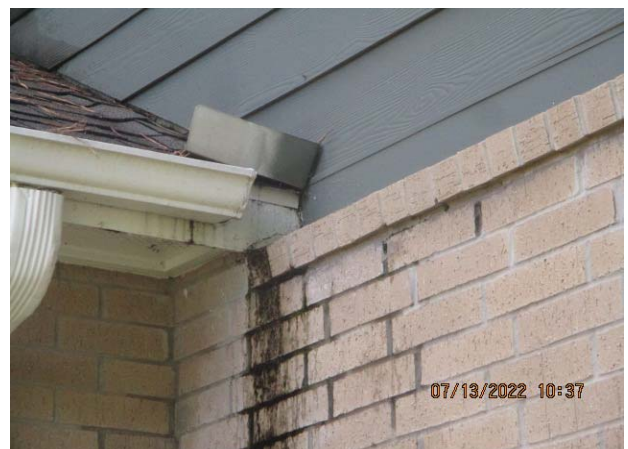
28. BUILDING 6: WATER FLOWS BELOW SHEET METAL WATER DIVERTER
