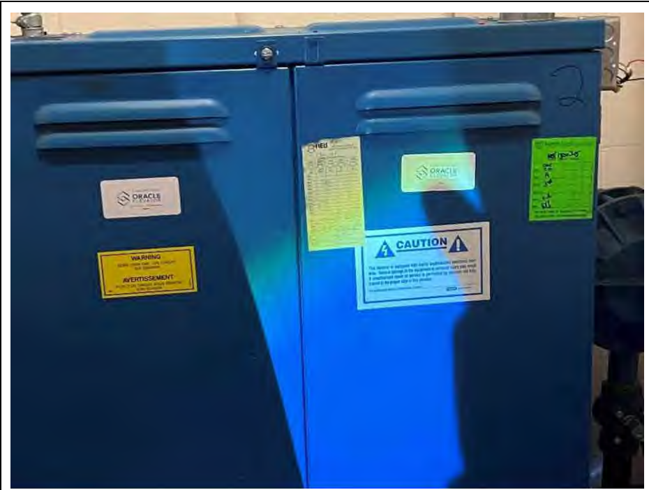
PHOTO #19 DESCRIPTION: Mechanical room to control the elevator (inside new addition of the church)
