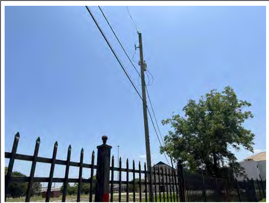
PHOTO #6 DESCRIPTION: Pole-mounted transformer (good condition)
