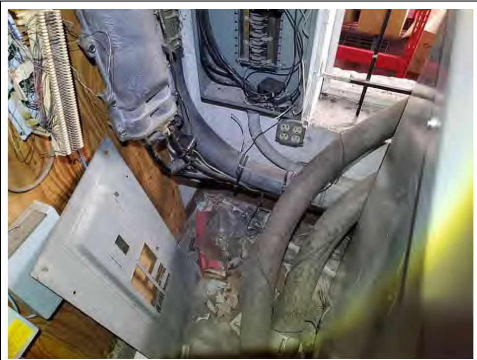
PHOTO #43 DESCRIPTION: Electrical room in original church
