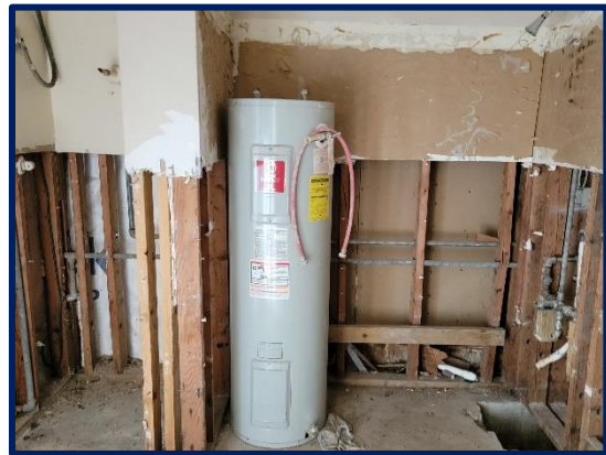
Vacant damaged unit
