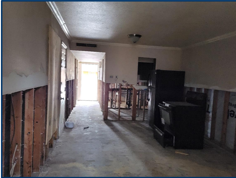
Interior view of one of the vacant units. All other vacant and damaged units are assumed to be in similar condition
