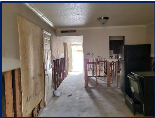
Vacant damaged unit
